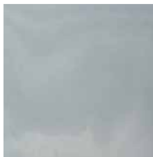
Weathered Concrete Ref: 92
